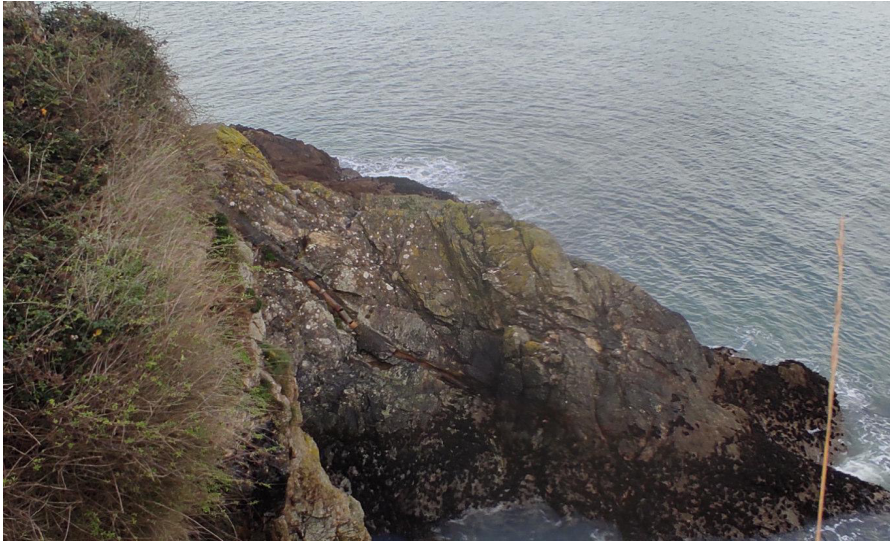
Figure 3: Sea Outfall Pipe
